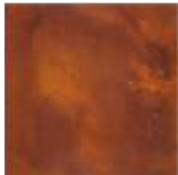
rust (beton powlekany)
